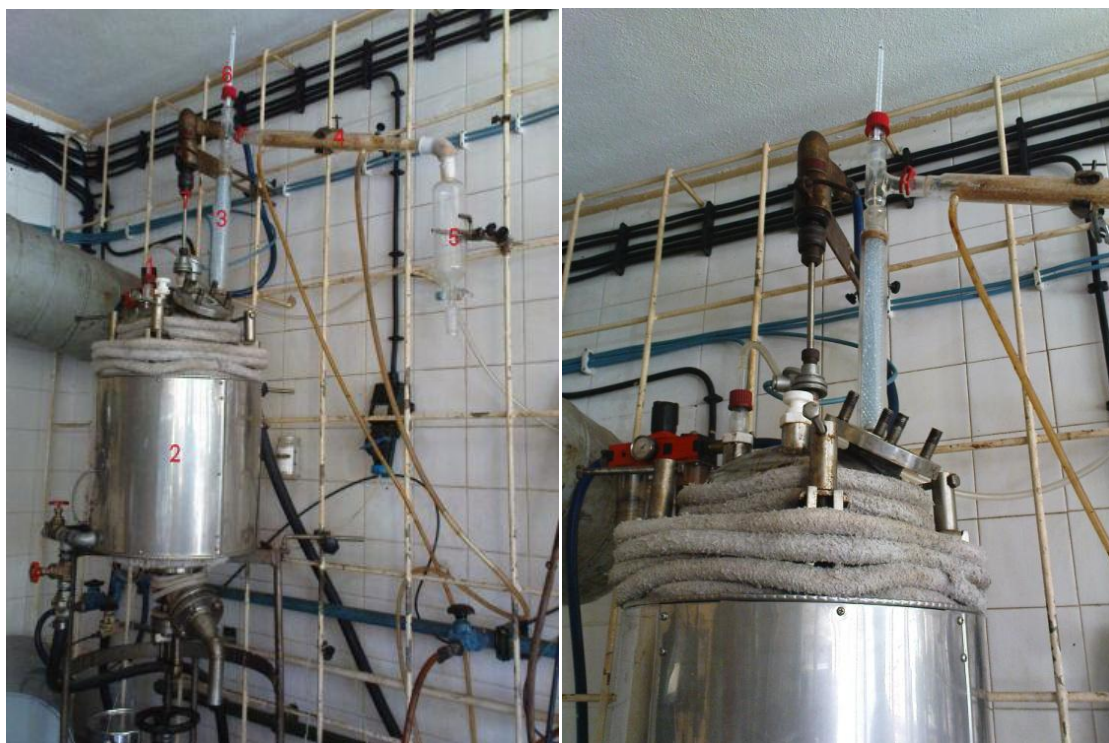
Figure 18: Pilot reactor at CPB. General view.
