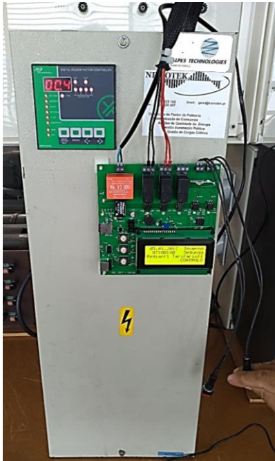
Fig. 19. – Device on the capacitor bank.
