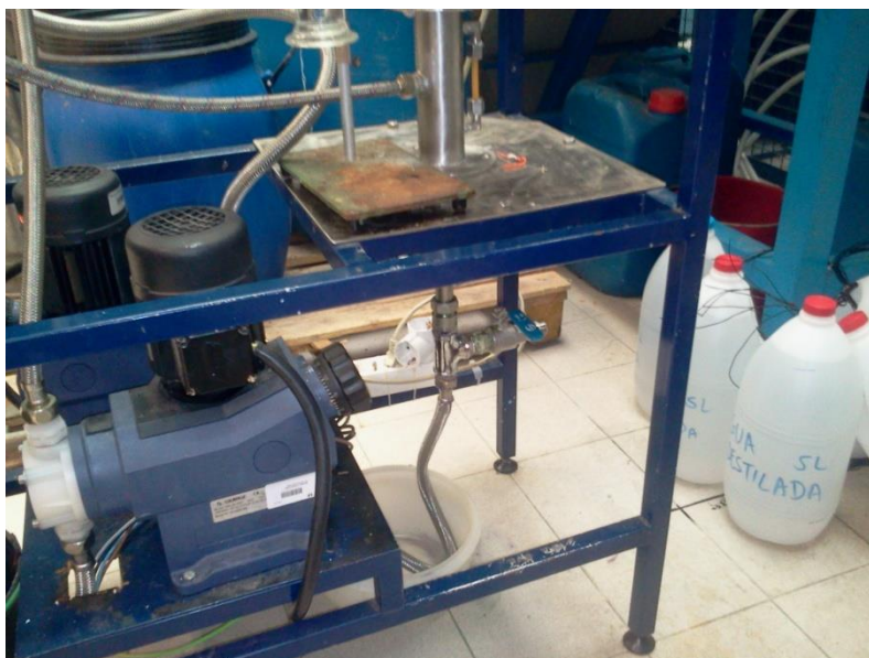
Figure 21 – Sampling valve downstream of the absorption column.
