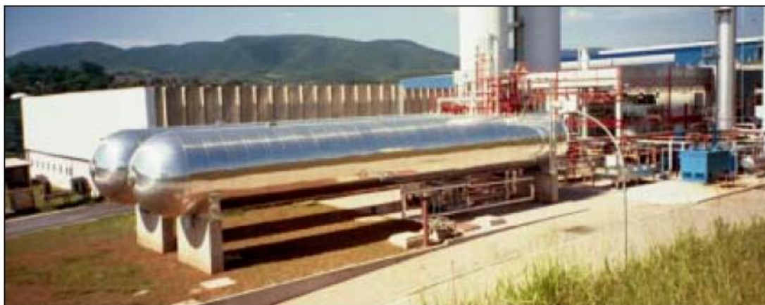
Figure 7 –Purified and liquefied CO 2 storage tanks in the Coca-Cola factory in Jundiaí, Brazil. [16]
