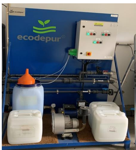
Figure 32: Enzymes dosing system
