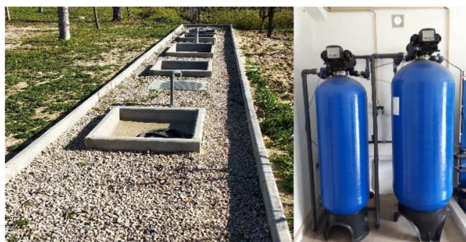
Figure 1. Wastewater treatment plant for Carwash (left: overview of the treatment plant, right: pressure filters)
