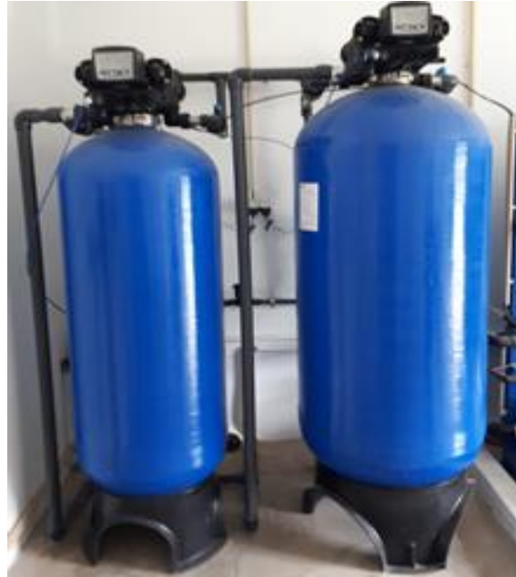
Figure 33: Pressure filtration system
