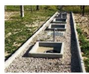
Figure 2. Wastewater treatment plant for Carwash- overview of the treatment plant
