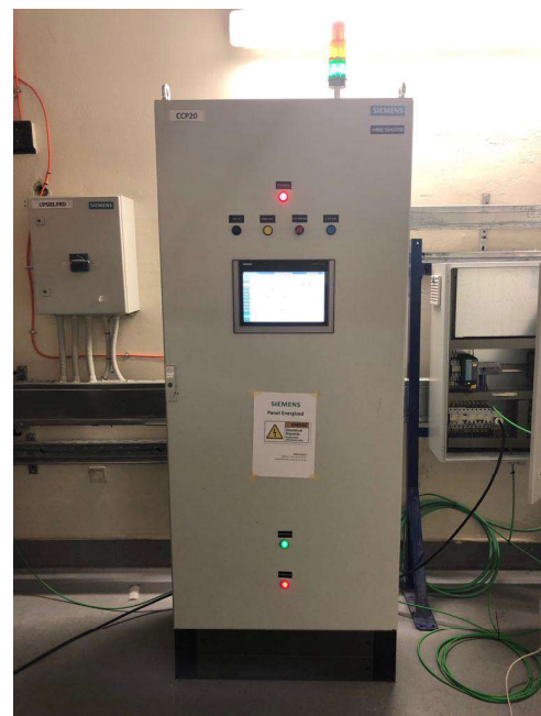
Figure C.2: Central Control Panel cabinet door.
