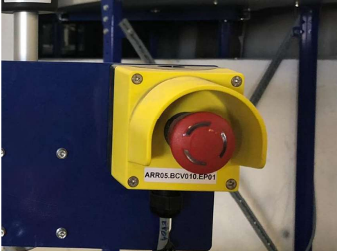
Figure C.12: Emergency Stop push button.
