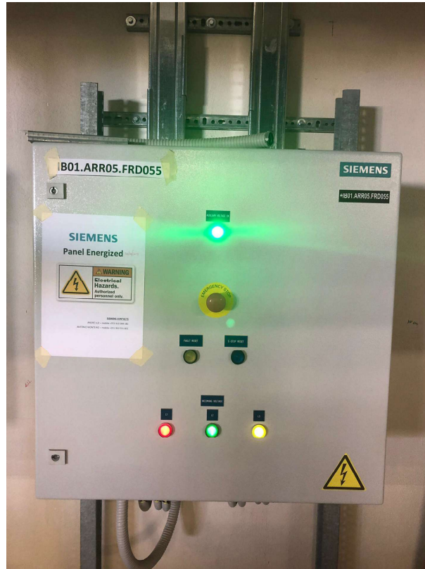
Figure C.6: Fire Door Cabinet.
