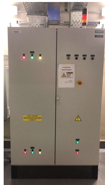
Figure C.3: Field Distribution Board.
