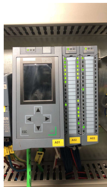
Figure C.1: SIEMENS SIMATIC S7-1516F.
