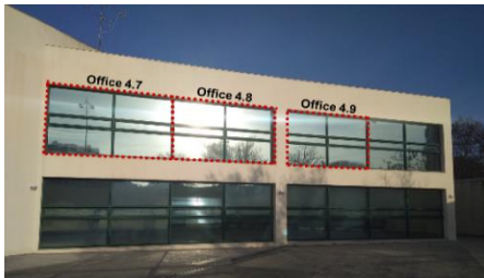
Figure 1 – Office’s glazing systems identified on the exterior façade (Southeast) of the building.
