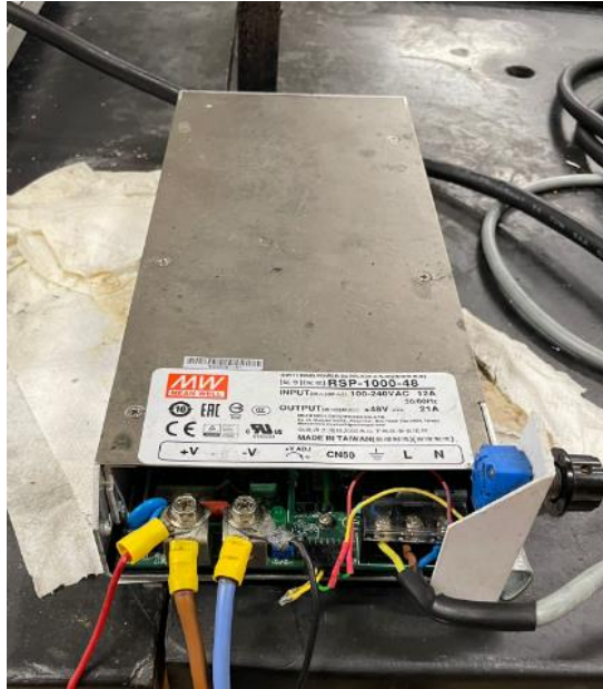
Figure 7-8: Power supply connected to the stack;
