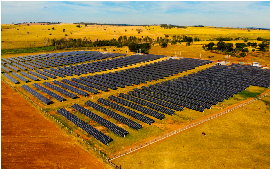
Fig. 1. PV plant layout with five modules, located at Loanda, Parana, Brazil.
