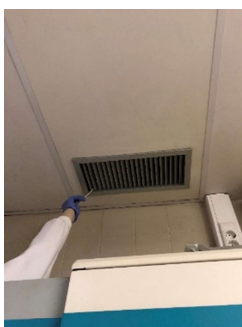
Figure 3.3 – Example of the swab's collecting in a ventilation grid
