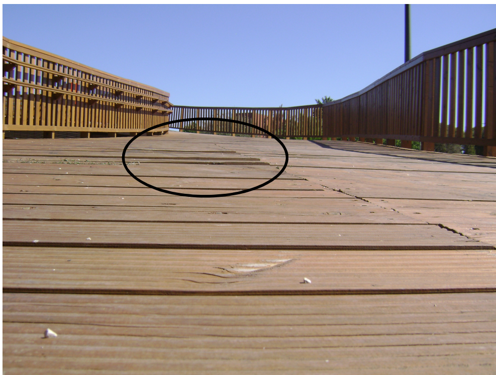
Figura 101 - Piso irregular (Almeida, 2013)
