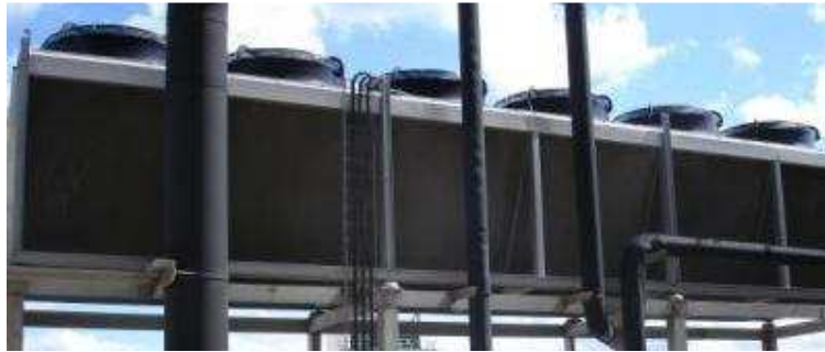
c - Dry Cooler / Air Blaster.
