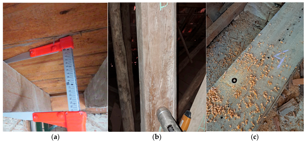
Figure 11. In situ inspection procedures (source: adapted from [33]). (a) Geometric survey of the timber elements; (b) resistance to penetration test; (c) core extraction.
