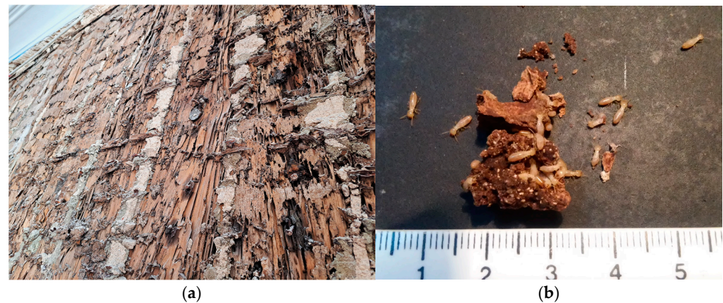
Figure 7. Appearance of wood degraded by subterranean termites (source: author's collection). (a) Decayed partition wall along its entire length after cladding has been removed; (b) Subterranean termite (removed from habitat) appearance and size.
