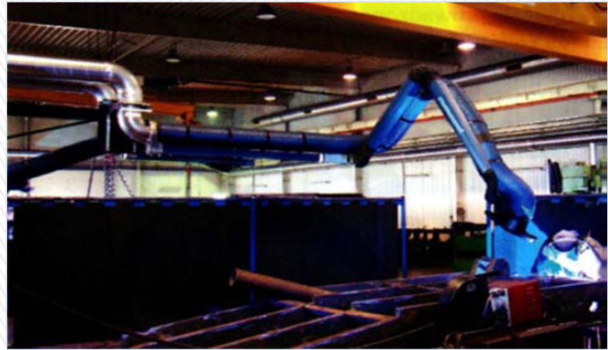
Rotating extraction arm suspended in order to cover a wide area of a welding workshop
